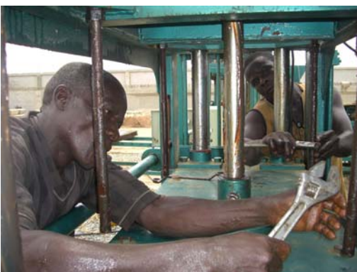
Installation in Africa
